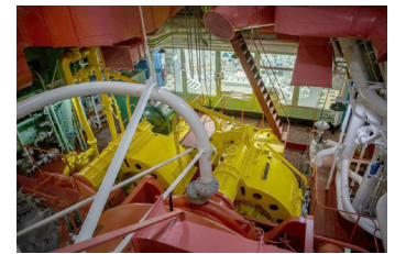
Engine Room/Reactor Compartment
